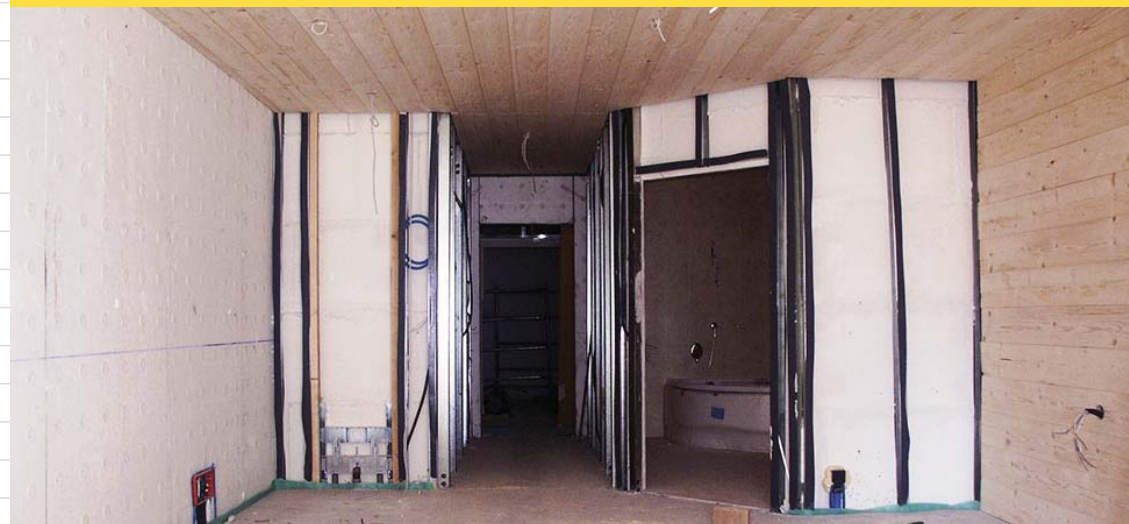
Wooden false ceiling
